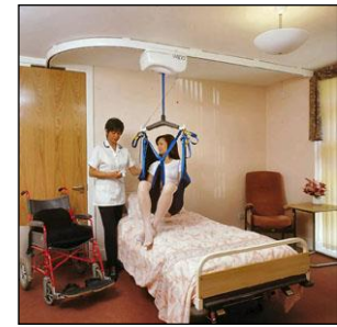
Figure 3: Ceiling Mounted Overhead Hoist
